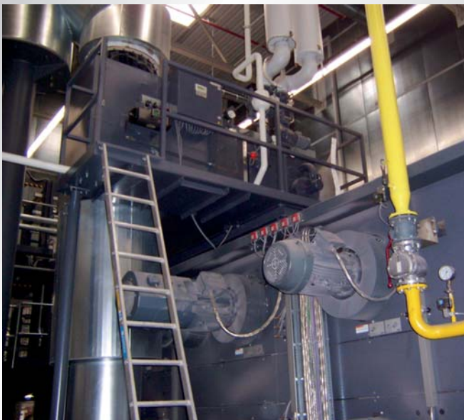
Heat recovery from exhaust gas from a drying kiln for the generation of heating energy.
