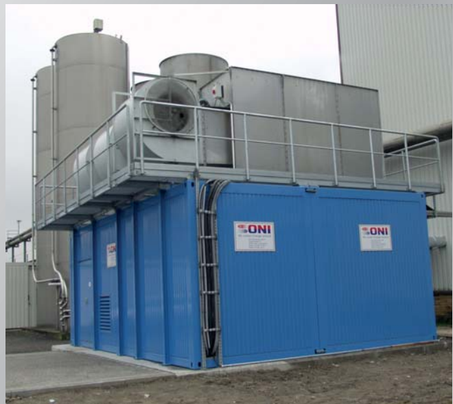
Energy-efficient container-based cooling system with hydraulically operated cooling tower recooling system.
